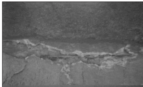
Major Damage to Fire Insulation
