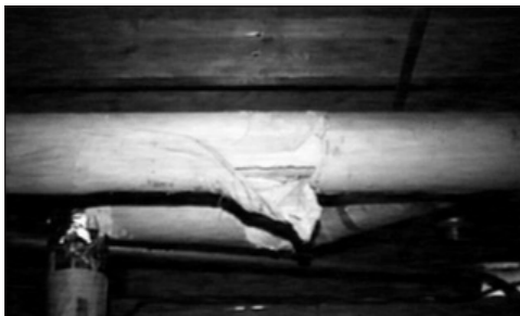
Minor Damage to Pipe Wrap
